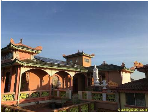
Solar system is installed on the roof top of one of Temple building
