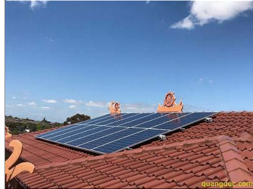
Solar system is installed on the side roof top of one of Temple building
