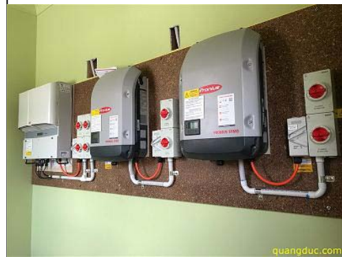
Two inverters of the 20kWp solar system
