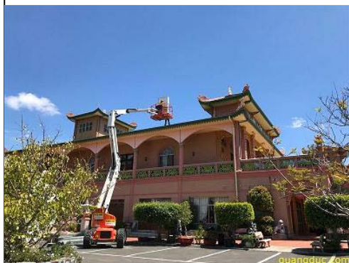
Solar installation is on the way to the roof top of the Main Temple building
