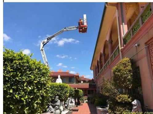
Solar installation with the help of a crane to reach the roof of a two storeys building
