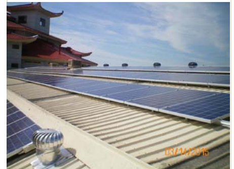
SOLAR PANELS TO THE COMMUNAL AND EATING HALL ROOFTOP
